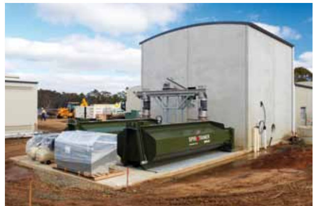
Dewatered sludge storage
