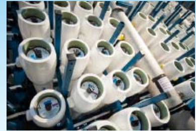
RO membrane racks
