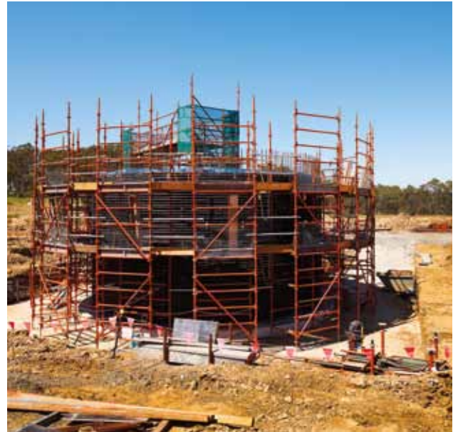
Digester under construction – the digester uses microorganisms to break down the biodegradable material. The gas produced through the process will be captured and used to generate heat for the digestion process.
