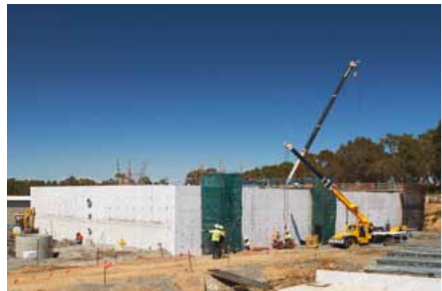
Bioreactor under construction – the bioreactor will be used to reduce the nutrients in the wastewater.
