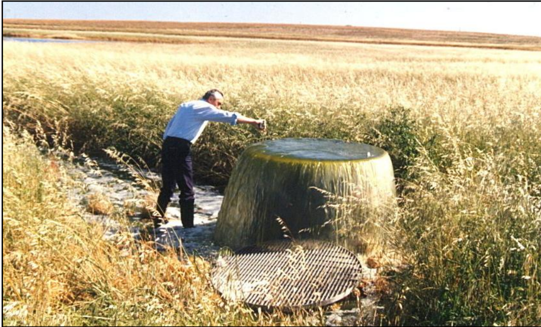
Figure 3.1 - The dissipator at the Murray Bridge WWTP Wetlands.
