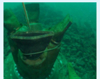
One of six diffusers on the outfall pipeline
