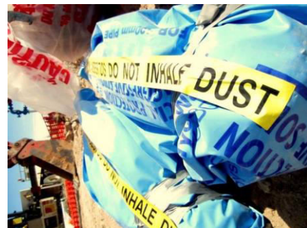
Photo 2: Double-wrapped asbestos material for temporary storage and disposal
