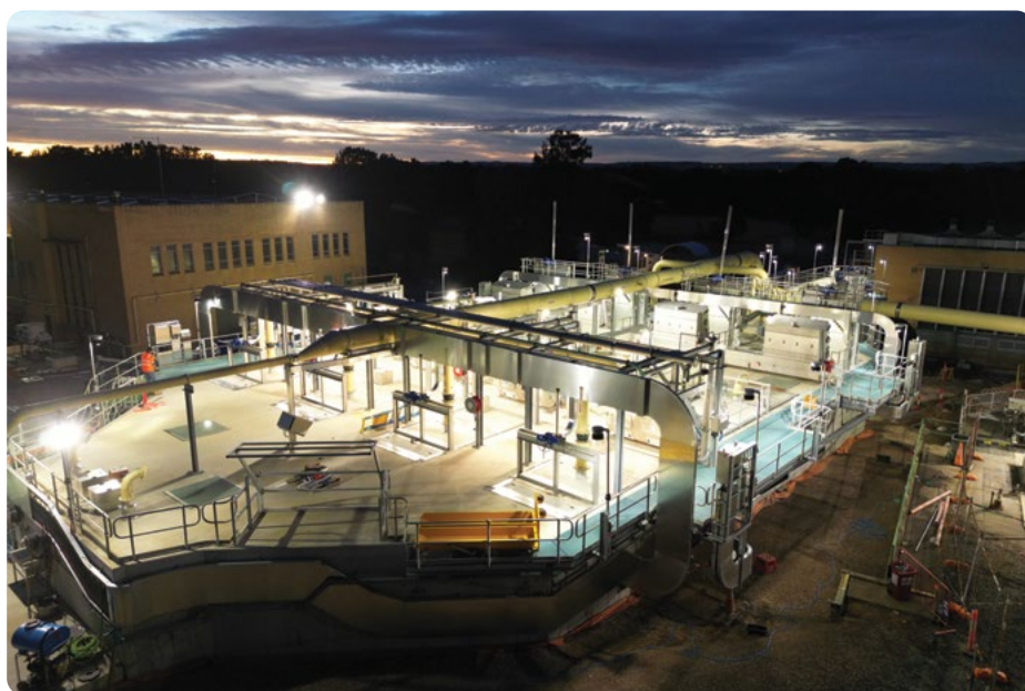
Bolivar's upgraded inlet structure is increasing wastewater treatment capacity to support Adelaide's growth.
