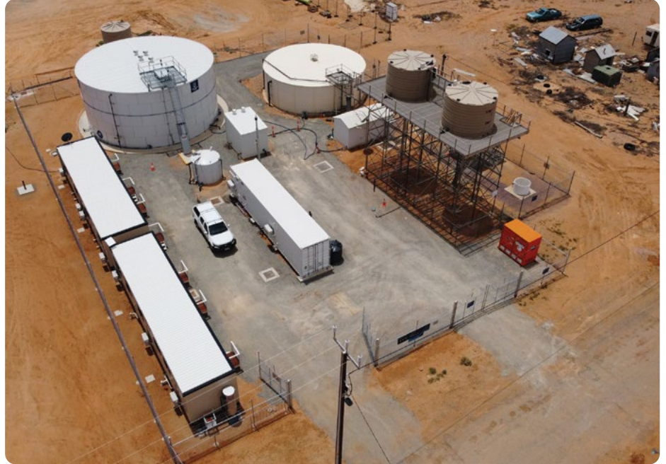
Marree now has access to safe, clean drinking water through its new desalination plant.
