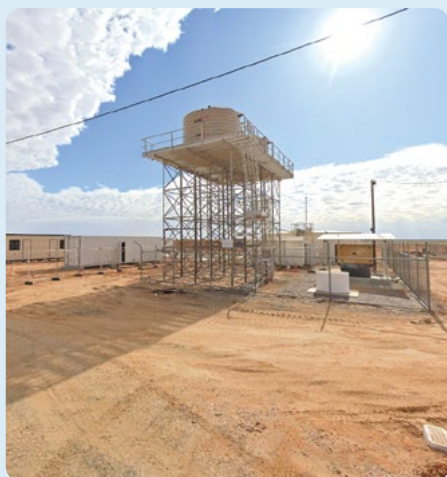
A new desalination plant commissioned at Marree is supporting safe and reliable drinking water supplies.
