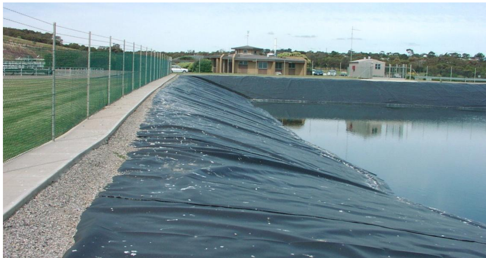
The treated effluent storage at Christies Beach WWTP. The fence has a concrete footing/path, but the liner is still simply returned into a backfilled trench. The aggregate is probably just a surface finish rather than the backfill. It is usual to try to avoid having sharp aggregates anywhere near a liner.
