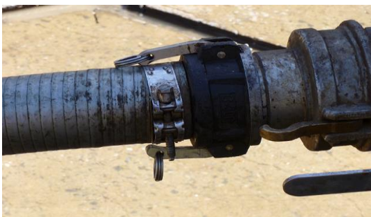
Figure 2: Cam-lock connection between tanker and SWDS discharge point
